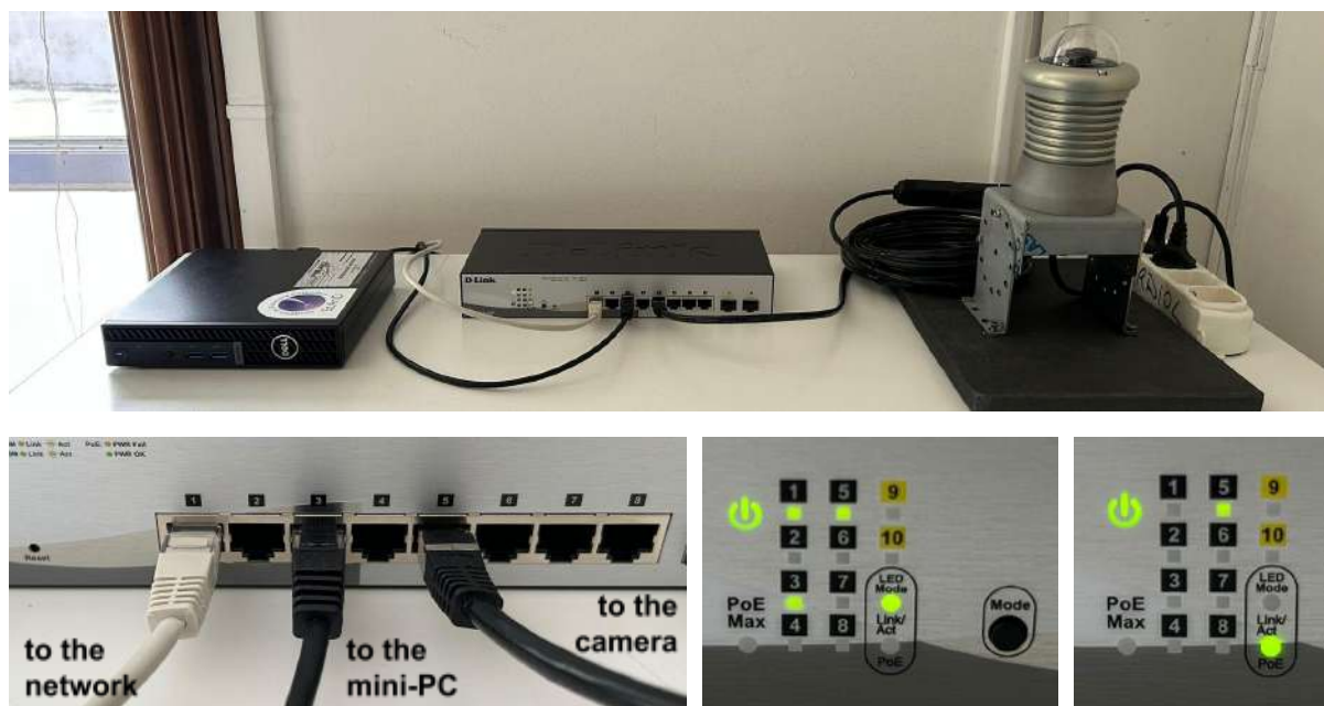
Figure 22 – Desk installation of the StAnd Meteor Camera Kit (top panel), picturing that the camera module is installed outside, and with connection specifics (bottom panels). For this installation, the Ethernet cables are plugged into the network switch as follows (bottom right panel). The Internet network is plugged in on port 1, the Ethernet cable from the mini-PC on port 3, and from the camera module on port 5. LEDs 1, 3 and 5 of the network switch are correctly lit up (bottom centre panel) and, when pressing the “Mode” button, only
